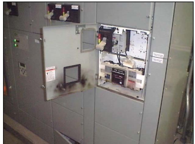
Switchgear Damaged By TVSS Unit Failure
